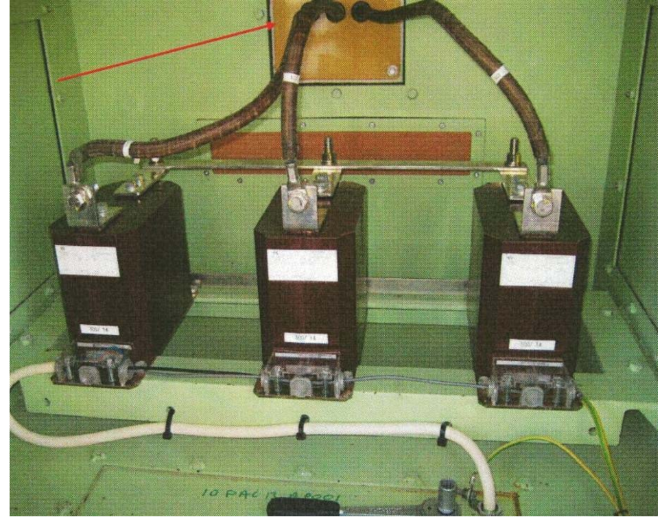
Image of winding connections. Neutral Cables and internal connections not spaced apart (arrowed)
