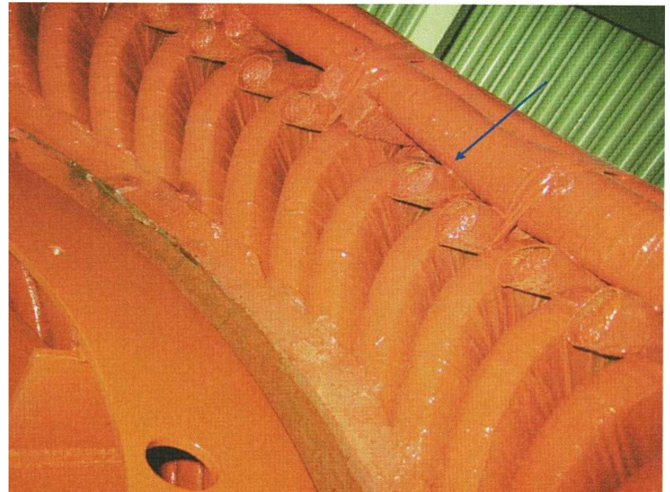
Image of coil – coil connections touching a neutral cable (arrowed) = design issue
