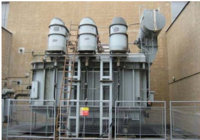
Power transformers and bushings
