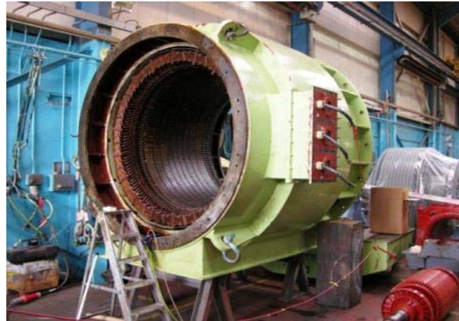
Motors and generators
