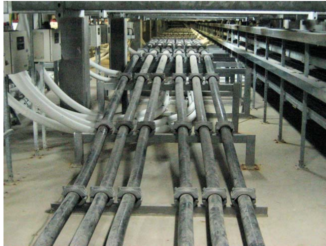
Power cables, joints/splices and terminations
