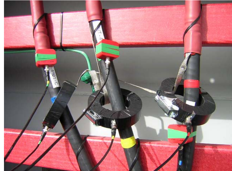
Sensor Connections at Transformer
