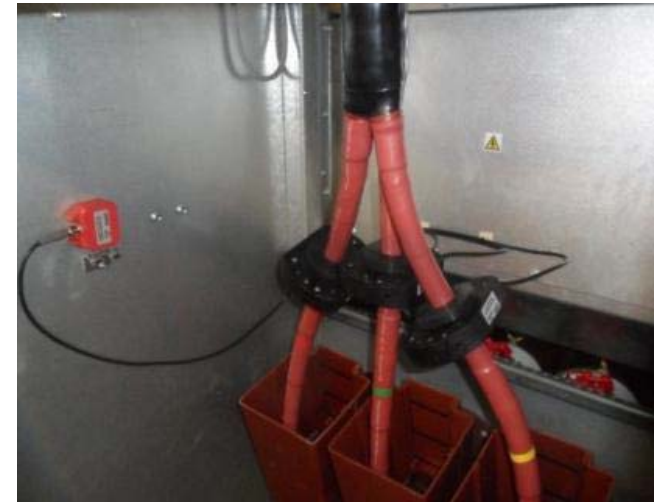
HFCT Installation (3) + 1x TEV inside an HV switchgear box
