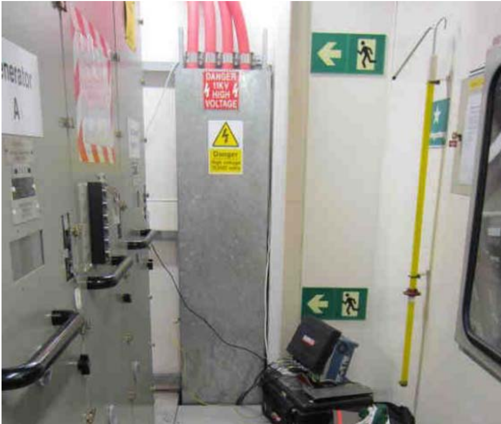
HVPD Longshot™ OLPD Test System at the 11 kV Switchboard
