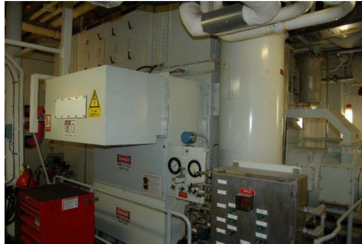
OLPD Testing of 6.6 kV Gas Turbine Generators (Cruise Ship, USA)
