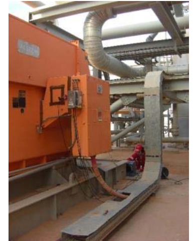
OLPD Testing of 10 kV Generators (Oil Processing Facility, Algeria)
