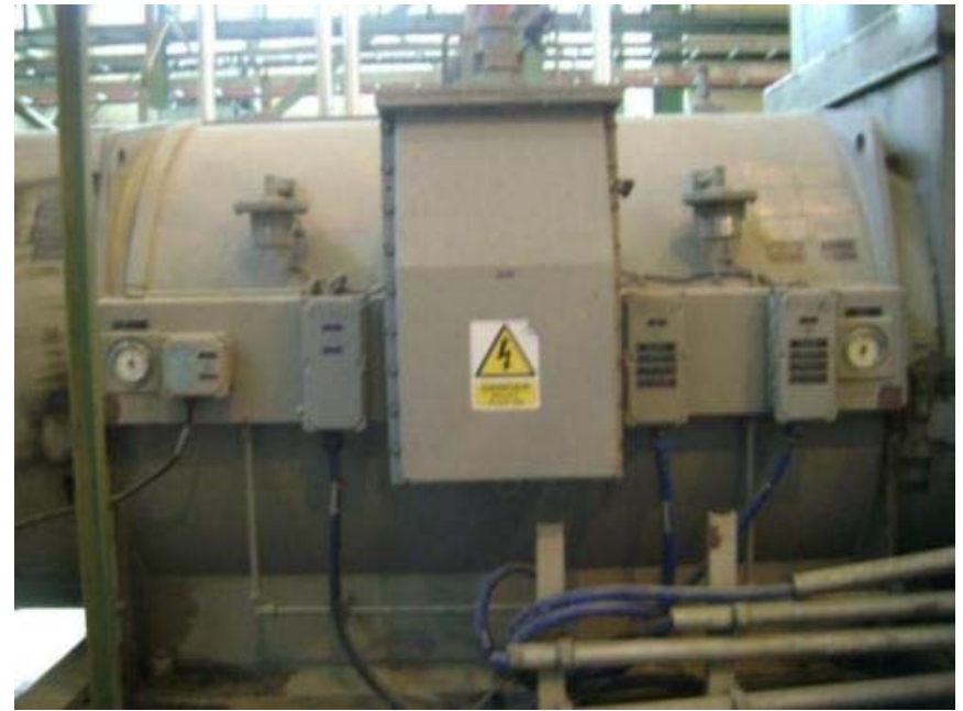
10 kV, 2400 kW Air Blower
