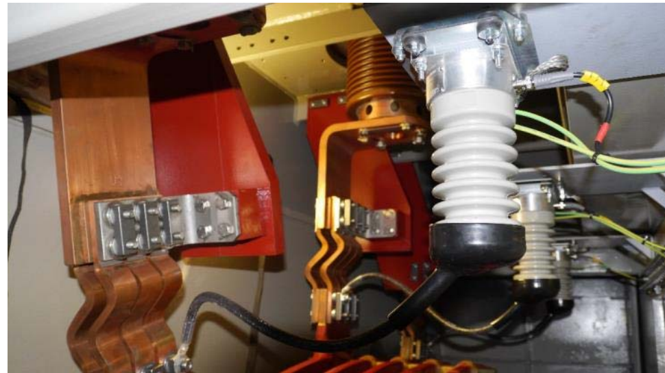
Example of a 15kV HVCC Sensor Installation (Oil Refinery, UK)
