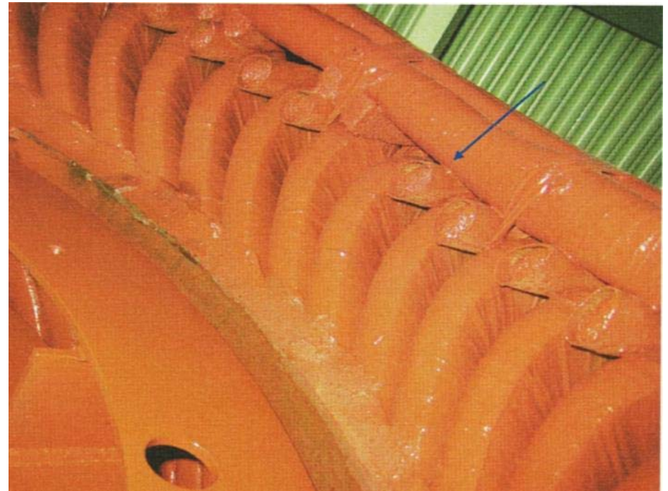
Image of coil – coil connections touching a neutral cable (arrowed) = design issue
