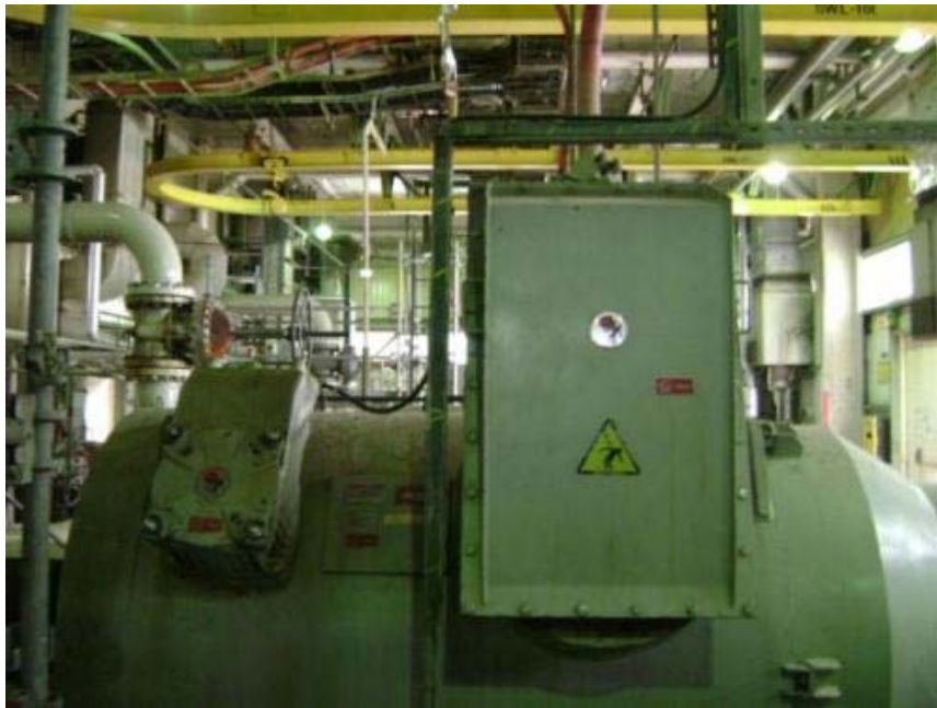
10 kV, 800 kW Amine Pump
