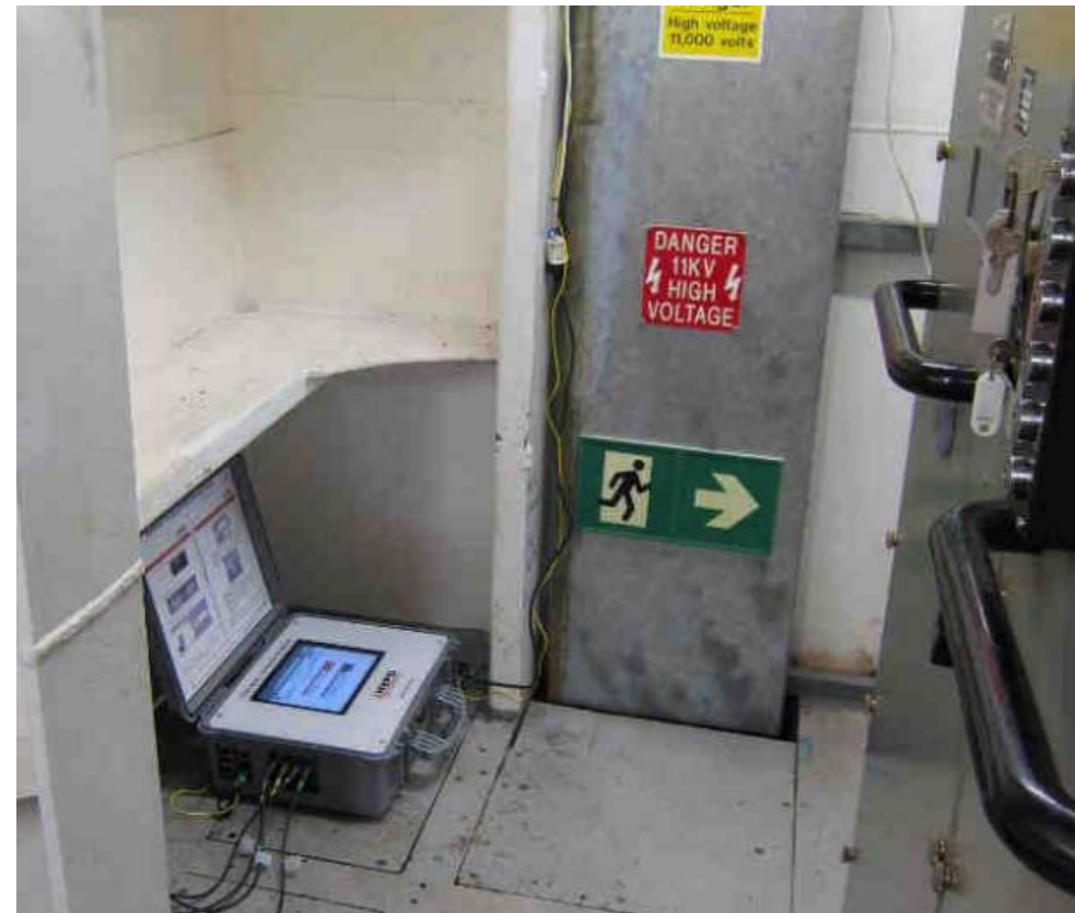
Portable HVPD Multi™ OLPD Monitor at the 11 kV Switchboard
