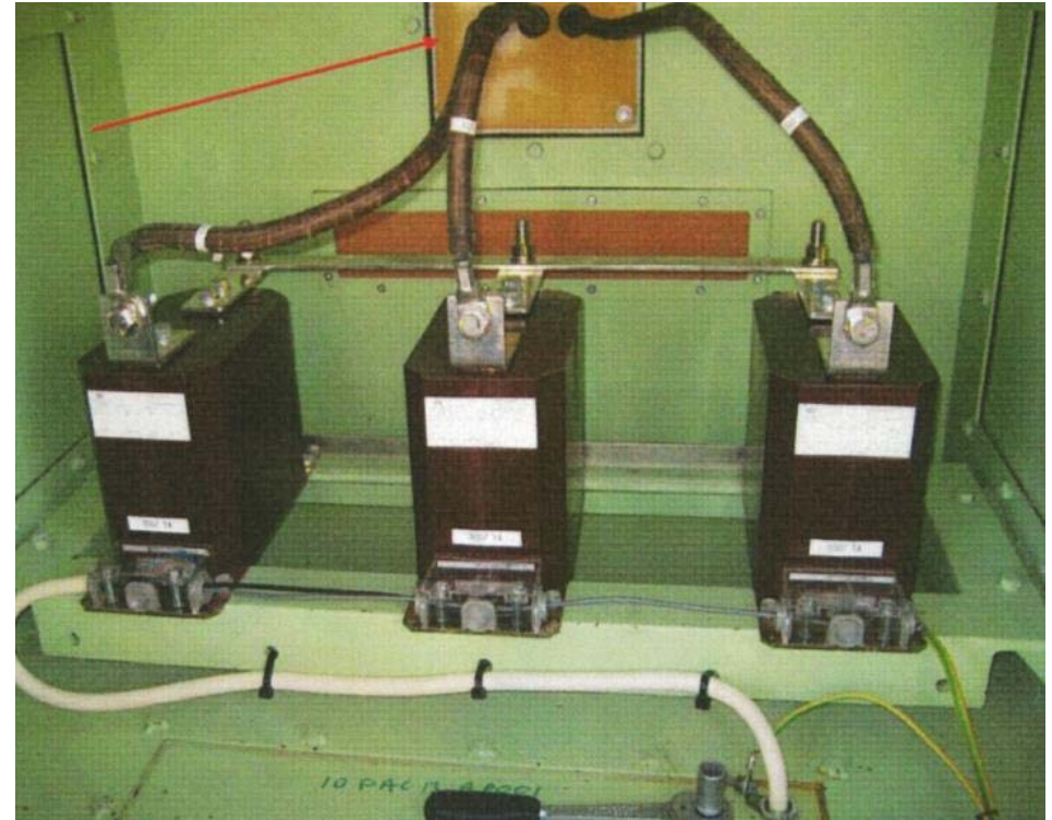
Image of winding connections. Neutral Cables and internal connections not spaced apart (arrowed)
