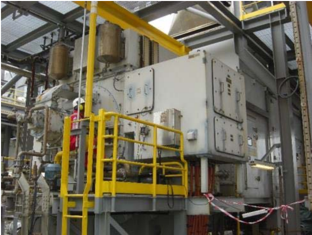
OLPD Testing of 11 kV GT Generators (Offshore Drilling Vessel, Angola)
