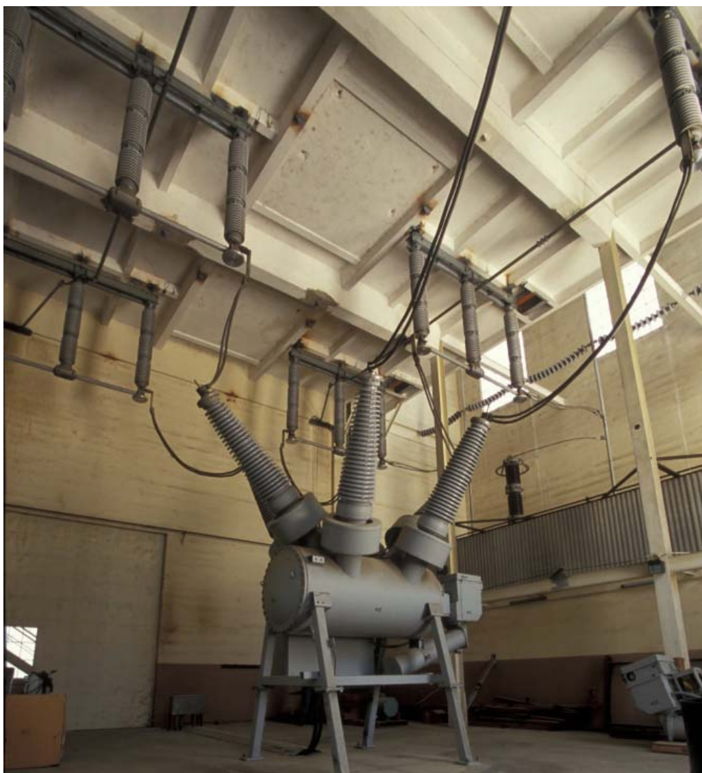
230 kV Indoor Generating Substation
