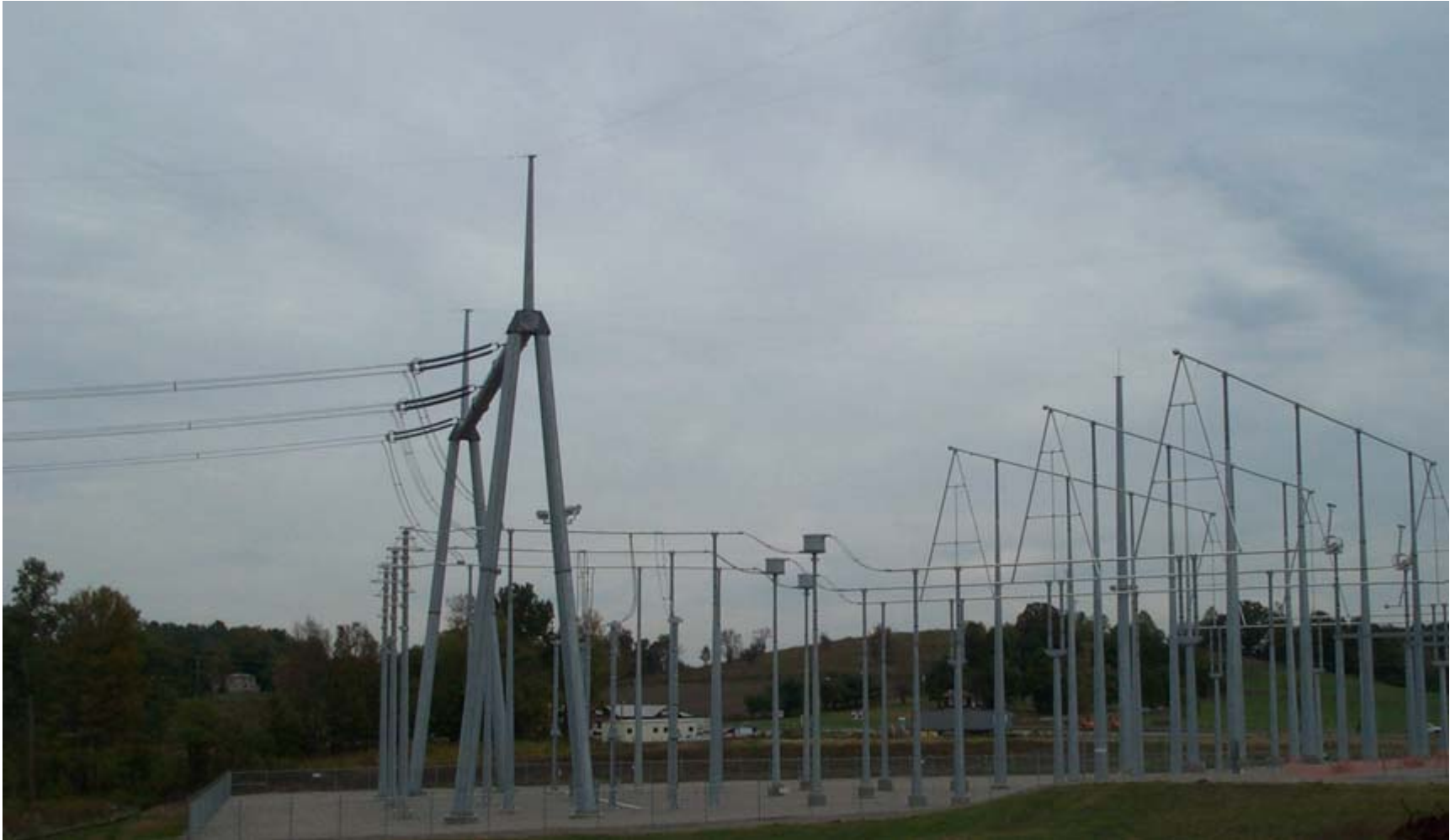
765 kV Generating Substation
