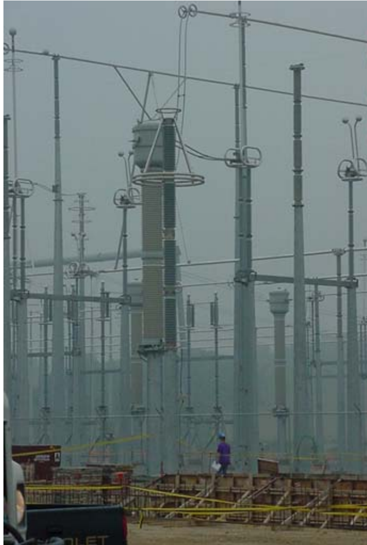
765 kV Generating Substation
