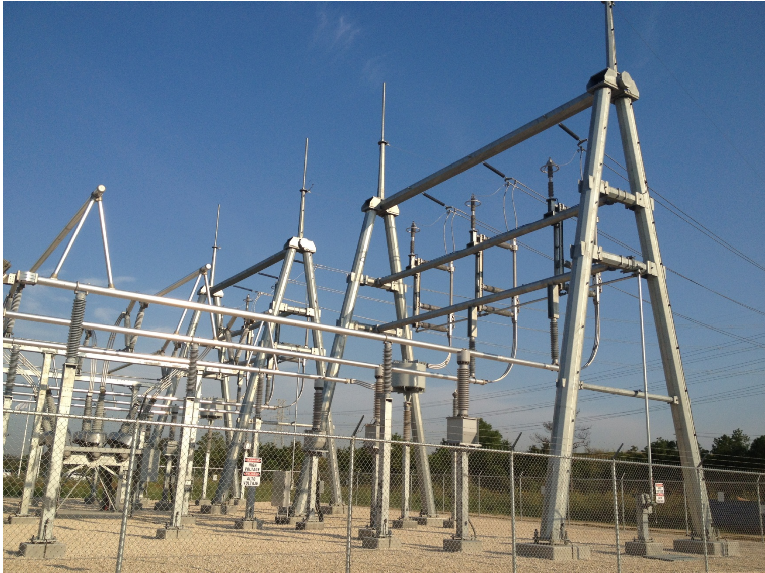
Typical 138 kV Substation
