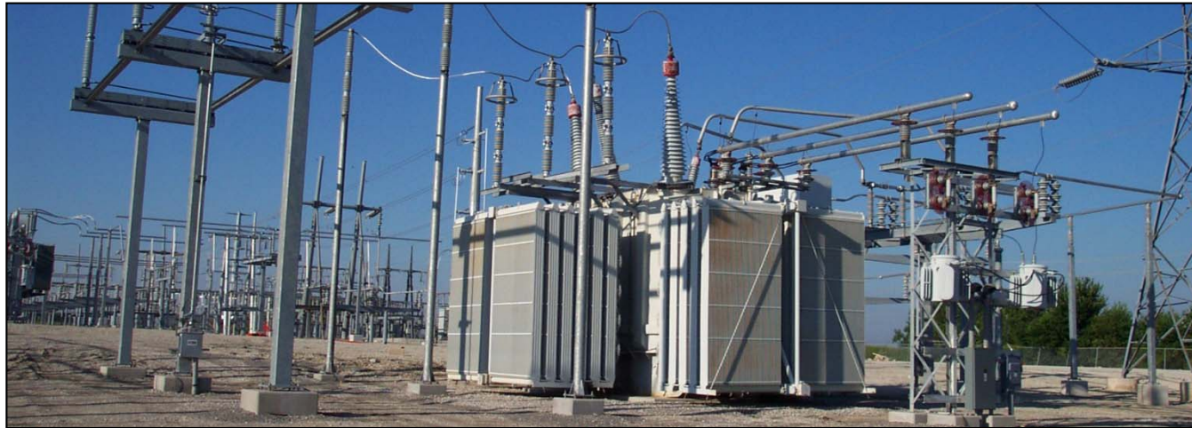
Relative Size of HV and EHV Power Transformers
