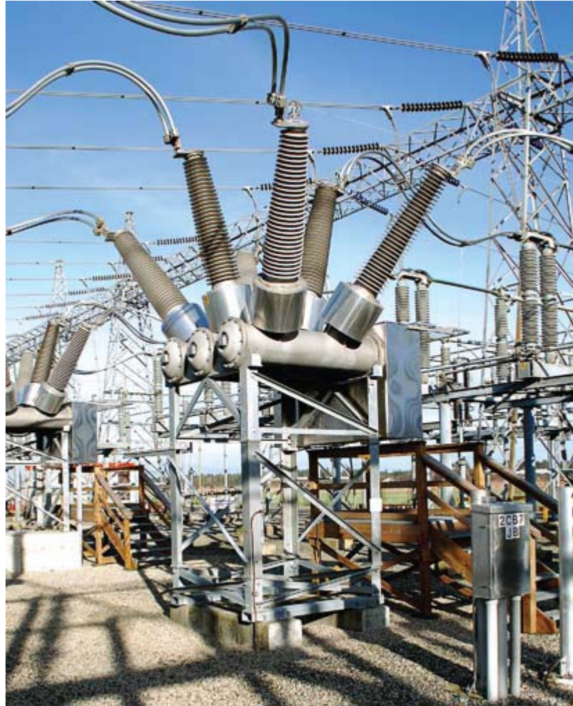
230 kV SF 6 Dead Tank
