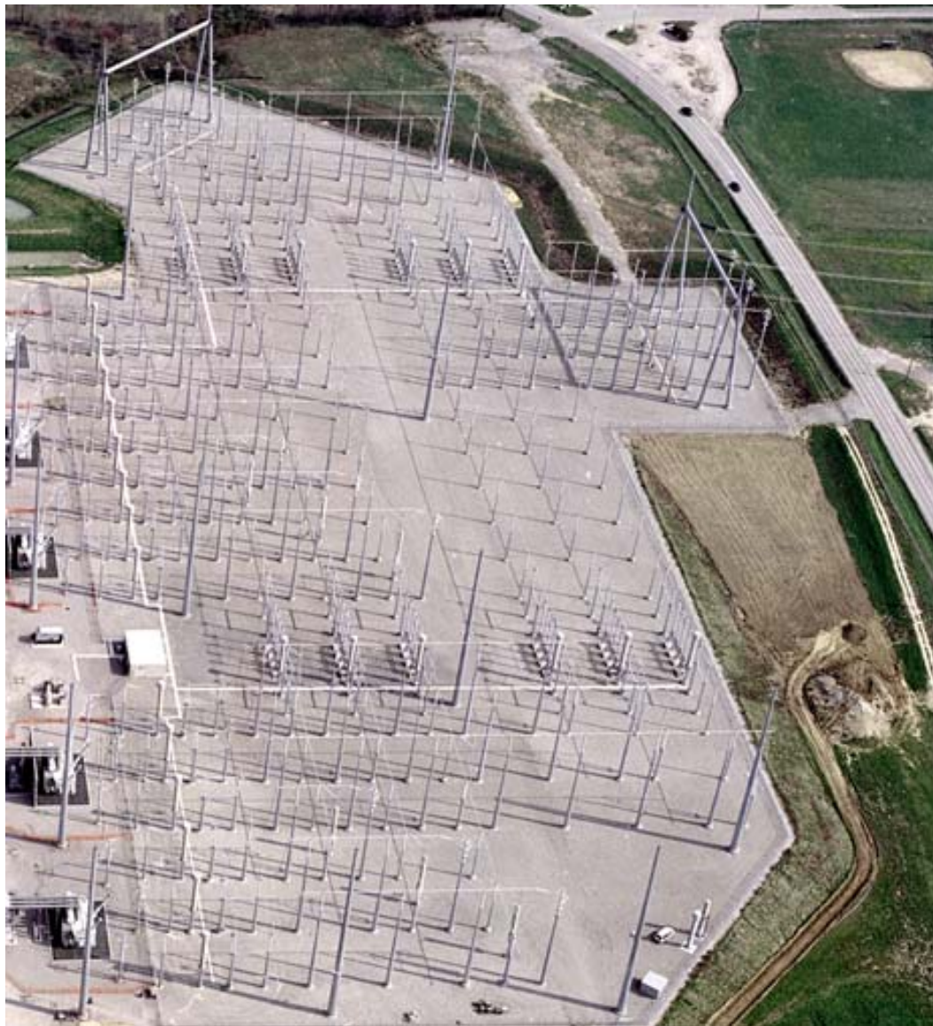
765 kV Generating Substation – Four (4) Breaker Ring Bus w/ Live Tank GCBs
