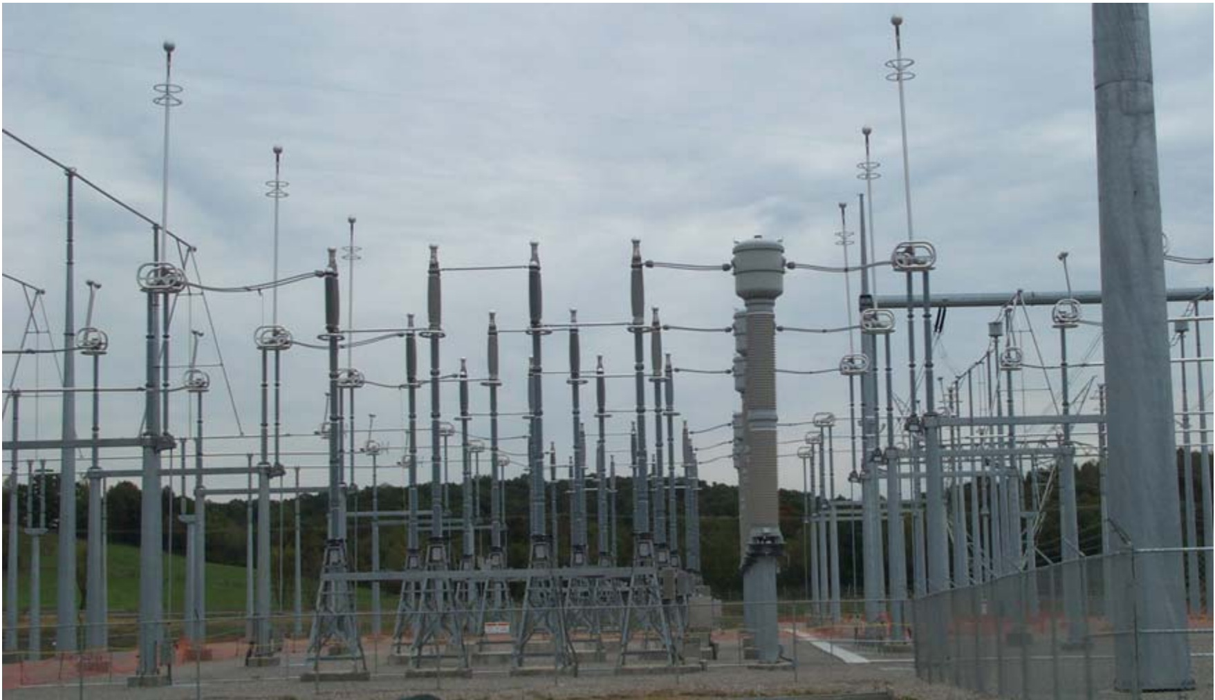
765 kV Generating Substation
