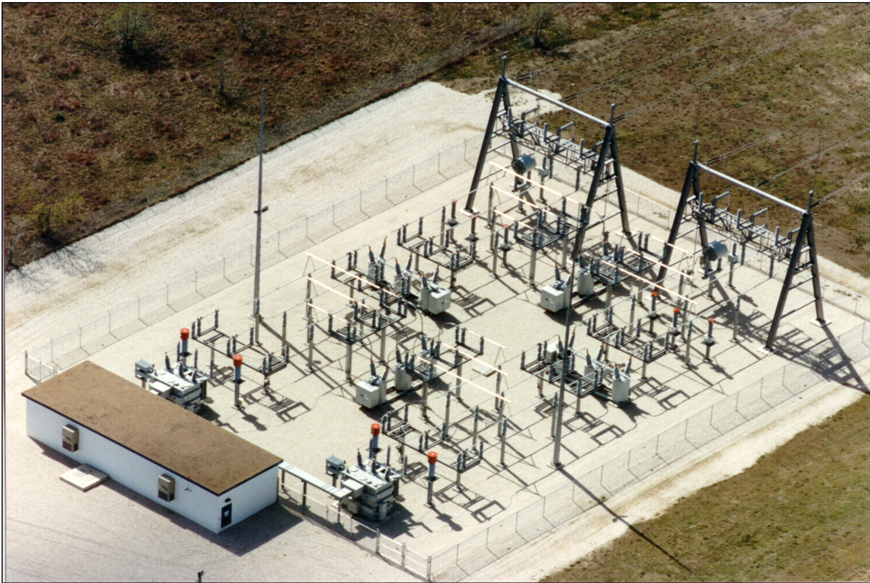
Typical 138 kV Substation – Four (4) Breaker Ring Bus w/ Oil Circuit Breakers
