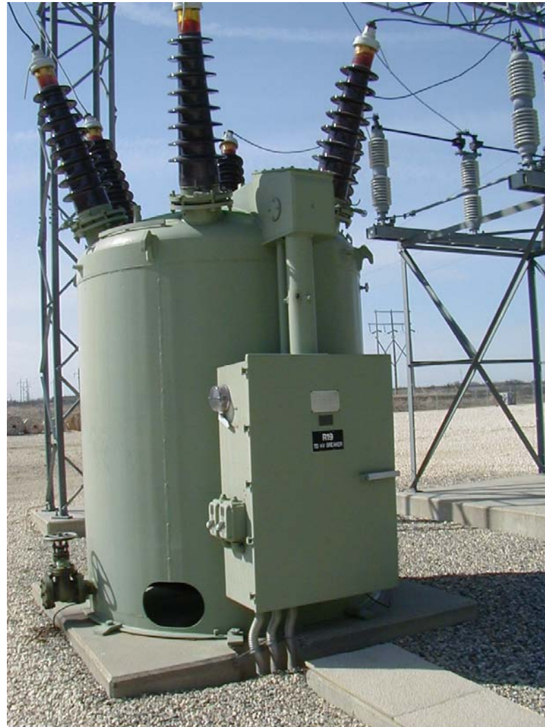
69 kV Oil Dead Tank
