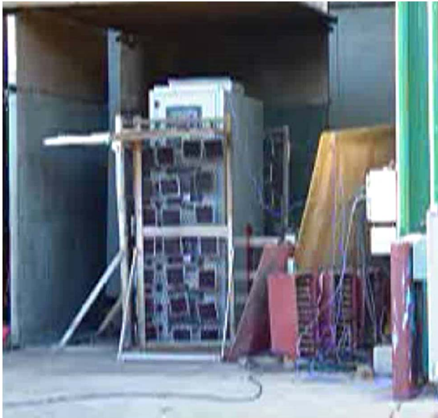
Solid grounded 3 phase 80kA .5 sec
