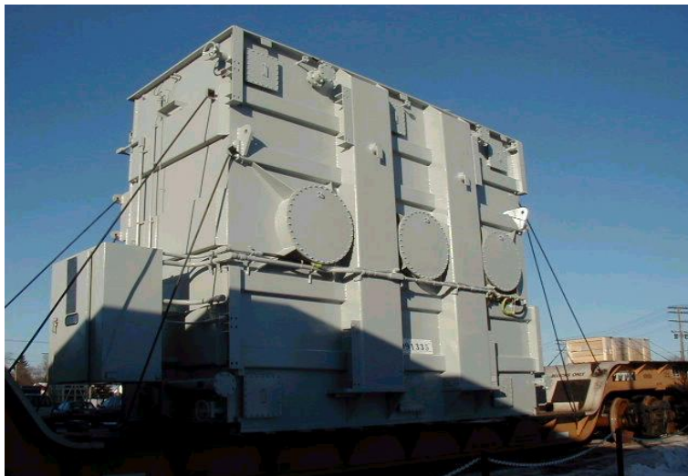
540 MVA, 345/22 kV GSU
