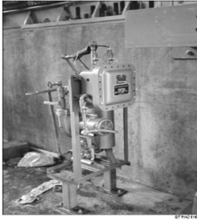
Figure 44. Hydrogen Dryer Used For 7FH2 Generator
