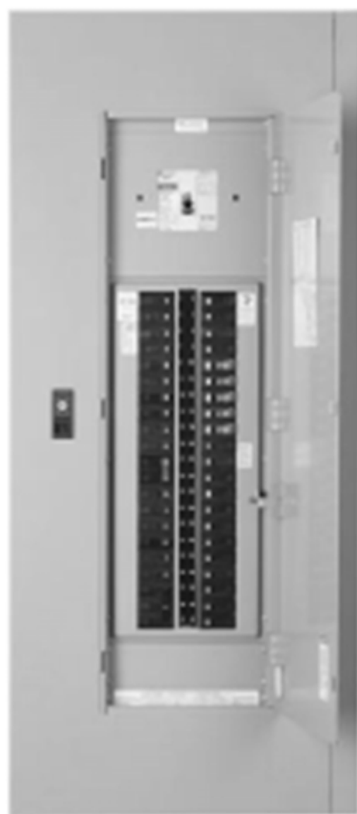
Type PRL 1a Panelboard
