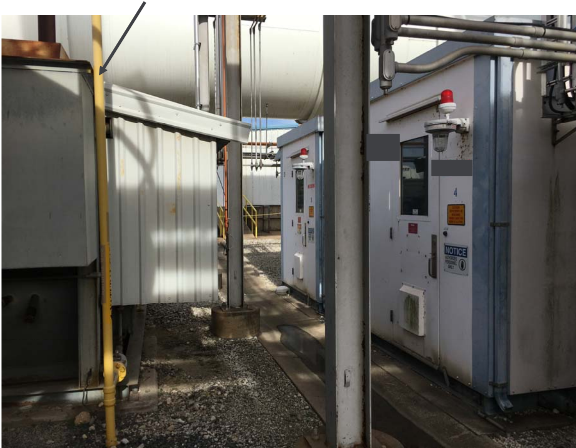
Natural Gas Piping
